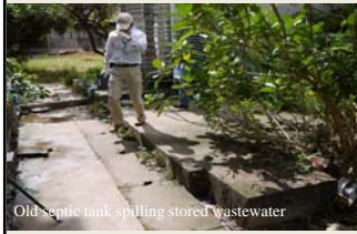
Old septic tank spilling stored wastewater
