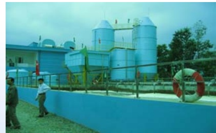
Nam Son Landfill leachate treatment system
