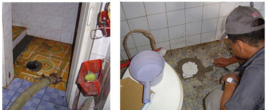
Worker installing plastic cover to the access hole after emptying septage in Hai Phong city Source: Author
