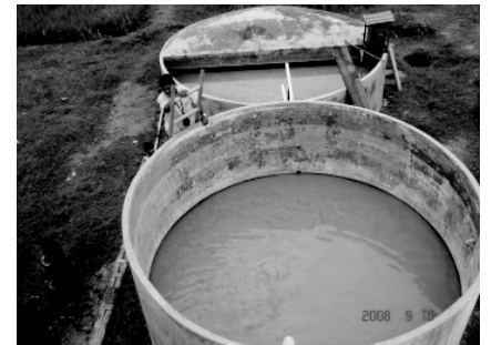
C.F.S. Tank and Slow Sand Filter
