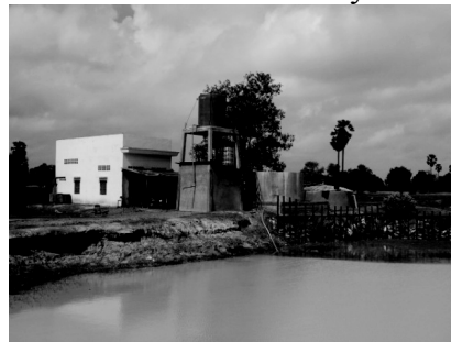
Water Treatment System
