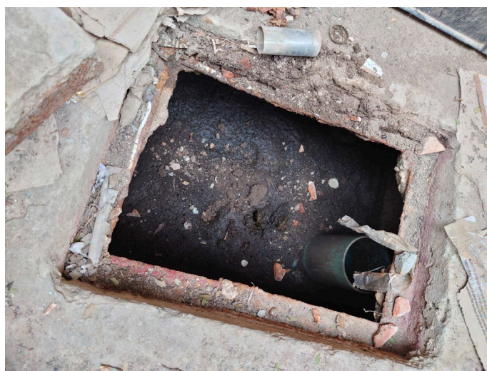
Figure 0.1-1 DEWATS filled with sludge due to lack of proper O&M
