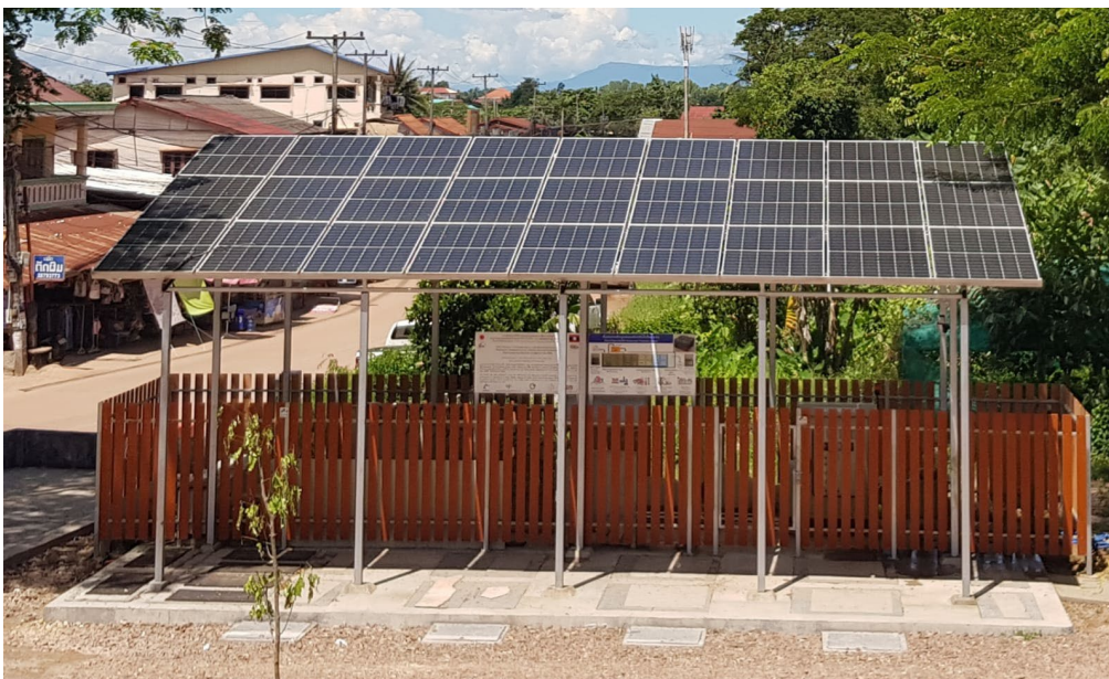
Figure 2.5-13 Wastewater Treatment System Utilizing Recycled Media KIDS with solar power at the Food Court of the National University of Laos
