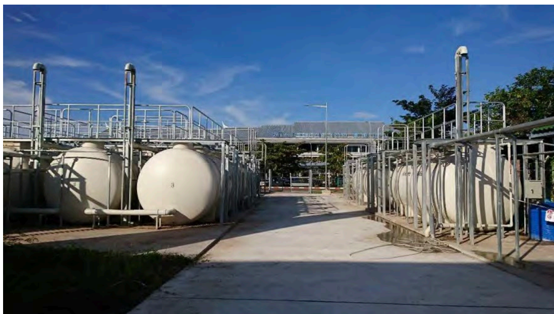
Figure 2.4-1 Johkasou system at Wattay International Airport (Kubota, 2022)
